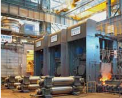
Arvedi ESP plant at the site of Siemens' partner Acciaieria Arvedi SpA.
